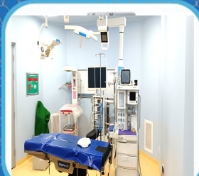
Modular operation theatre
